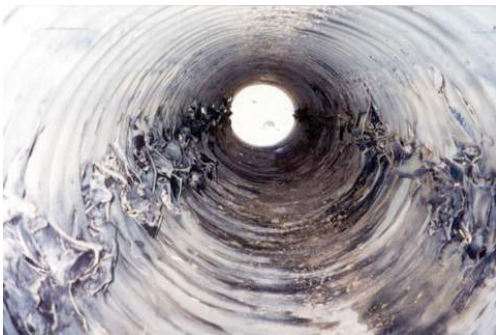
Figure 8 Wall crushing in geopipe
